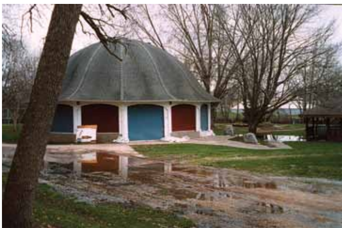
This is a photo of the carousel building after a typical spring rain taken in April of this year showing the standing water remaining around it. Peter and Leah Farnsworth photo
