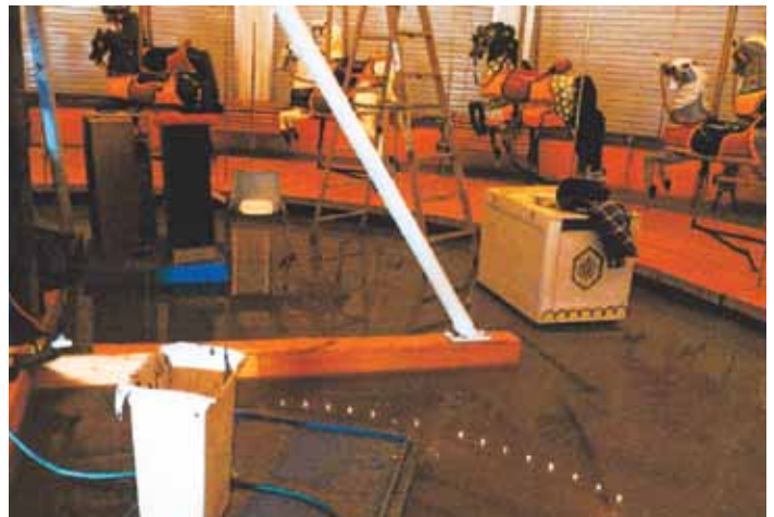
In this photo taken by Robert Hanson in June 2008, the flood waters had just begun to rise and now covered the floor. At this point the electricity in the building was still on and you can see the reflection of the lights above in the water below.
