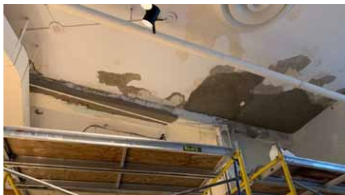
The Merry-Go-Round Museum fixed its plaster ceiling and painted the ceiling and walls to prepare for the new season.
